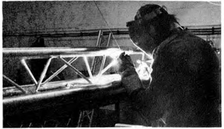
Ray Turner at work welding spars in a 5m length of Trilite. Aluminium welding requires both special skill and equipment.
